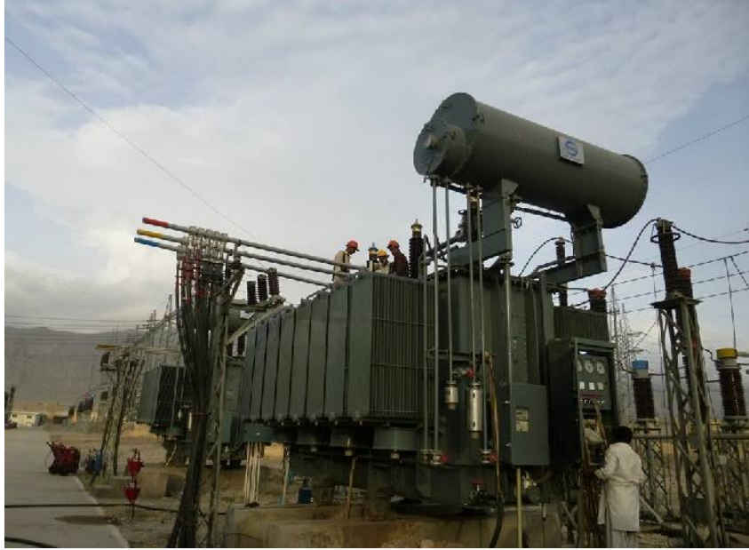
Augmentation at Quetta Industrial Grid station
