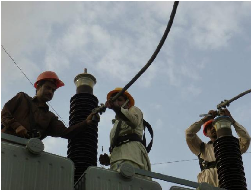
Augmentation at Quetta Industrial Grid Station
