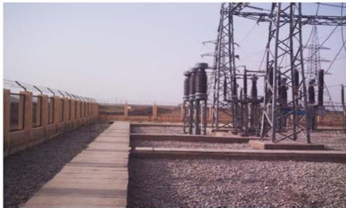
Open space at Yaro Grid Station
