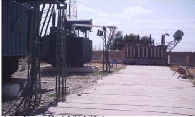
A view of the yard of Qila Safiullah Grid Station
